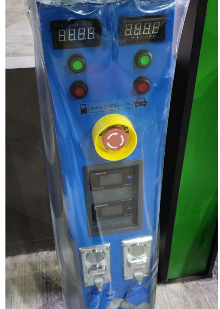
Charging station in a dedicated parking slot
